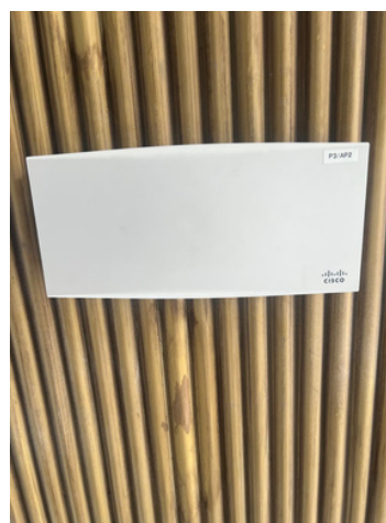
Cobertura WiFi Interior
